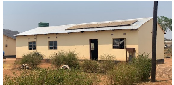
Dining Room Solar Panels
